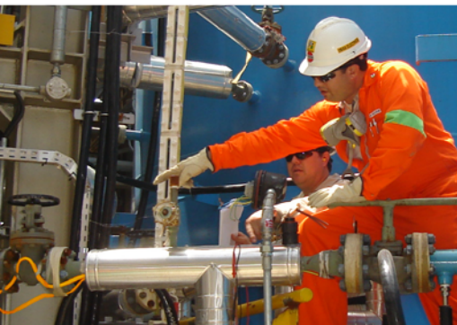
PIPE AND VESSEL HEATING
